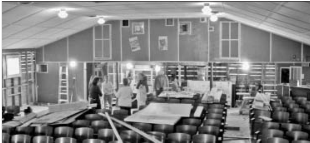
It's difficult to remember the abandoned and deteriorating state the theater was in, in 1999—with daylight coming through the walls during restoration work, above, and the need to clean out a family of raccoons and lots of debris. Among the work done: rebuild the northwest corner of the building; install two new, handicapped accessible bathrooms; create a fire exit to meet local state codes; reshingle and reroof the entire facility; install steel girders in the historic fly; build a public-access community walkway and completely insulate the theater and install an energy-efficient heating system to allow year-round programming. Photos courtesy of Opera House Arts
